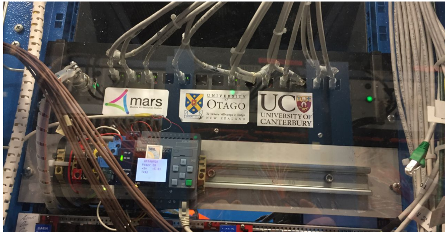
Readout chassis in Underground service cavern (USC) at -87m
