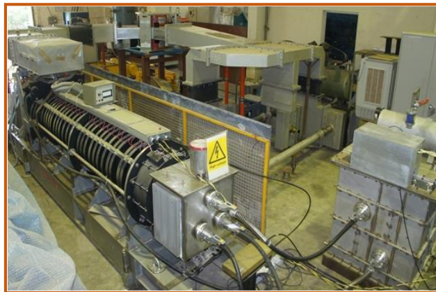
CERN klystron and circulator tested at 1MW peak power at RRCAT test stand.
