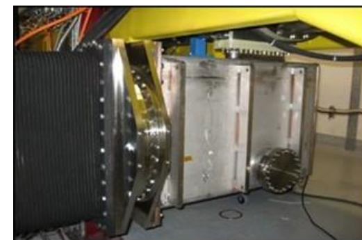
Two Cu coated SS WR 2300 waveguide power couplers installed in the DTL/CCDTL in LINAC 4 tunnel at CERN
