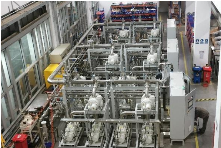
Cryogenic system hall in Jan. 16, 2020
