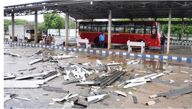
Damaged bus stop due to TC Mandous, HT (online), Dec 11, 2022
