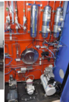
Closed loop gas system
