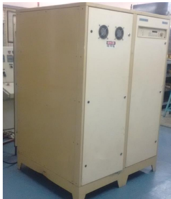
Magnet power supply 30V DC, 1200 AMP
